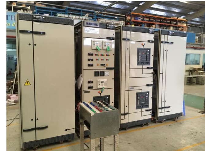
Center control PLC cabinet
