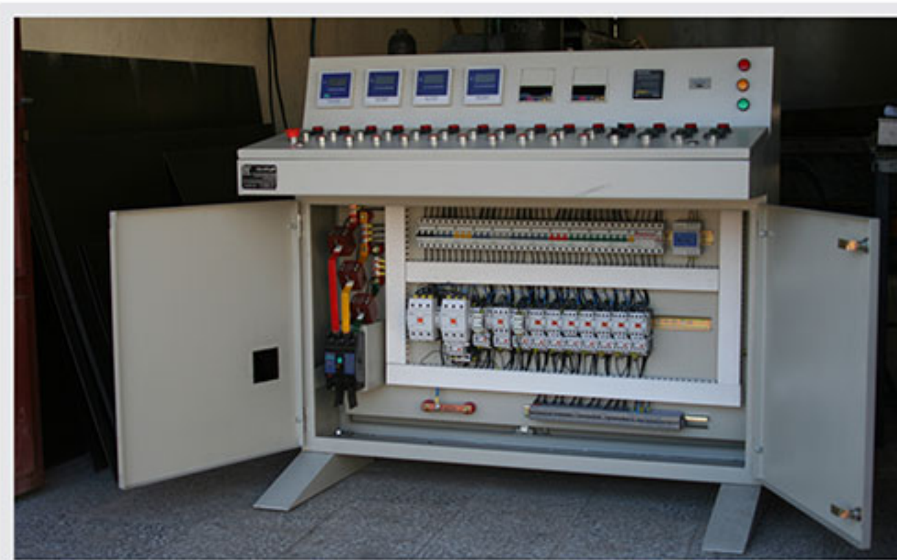
Central Control Panel
